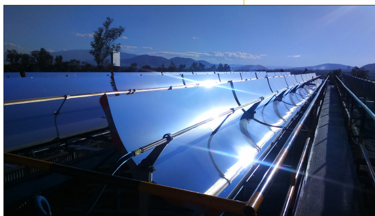
▲ Parabolic troughs used for preheating water at a tequila plant in Guadalajara, Mexico, installed by Inventive Power. (Photo credit: Inventive Power)
