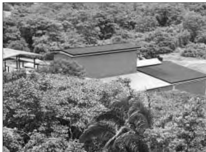
Solar system on a coffee drying plant in Panama. The system preheats air before it goes into the furnace. In this case, the objective is to reduce the amount of firewood used, but the system can also be used on other plants in the country,
