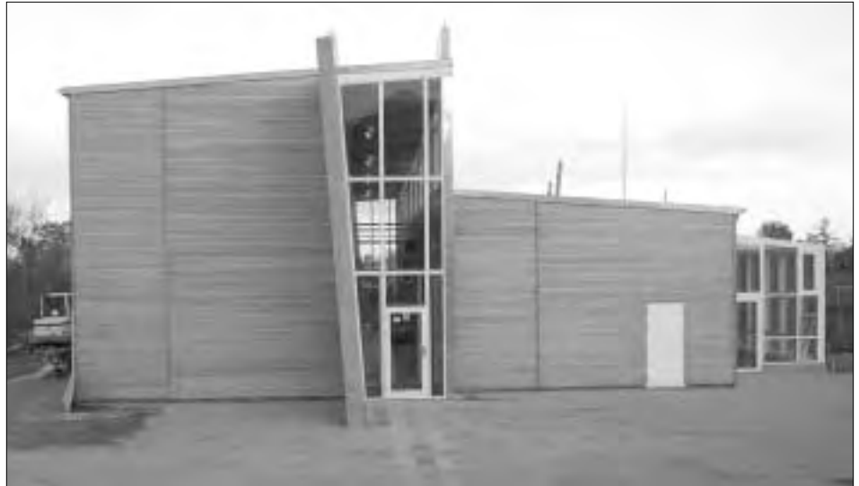
The first Task 23 demonstration project: Kvarterhuset community center in Kolding, Denmark, which is under construction.
