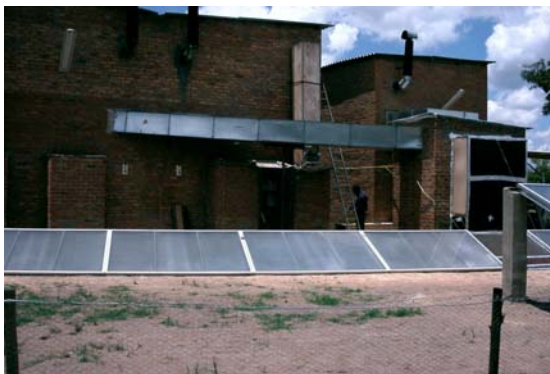
Tobacco drying facility in Zimbabwe.
