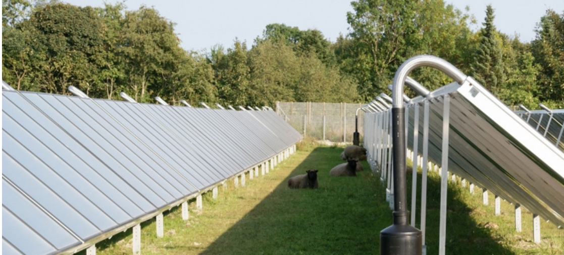
Figure 5: Ground mounted collector field at Trustrup-Lyngby Varmeværk. Source: ARCON-SUNMARK.
