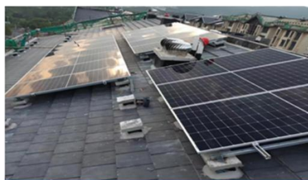
Solar energy project in Tianjin
