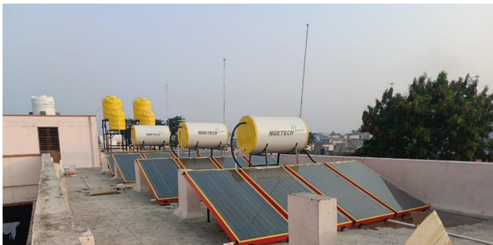
Figure 1. Thermosyphon System “Raichur Hostel for Girl Students”. Source: Nuetech Solar Pvt. Ltd.
