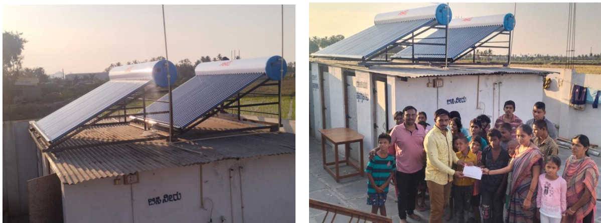
Figure 3. Installed Collectors at Government School Ballari (Karnataka State). Source: Jaideep Malaviya, Malaviya Solar Energy Consultancy
