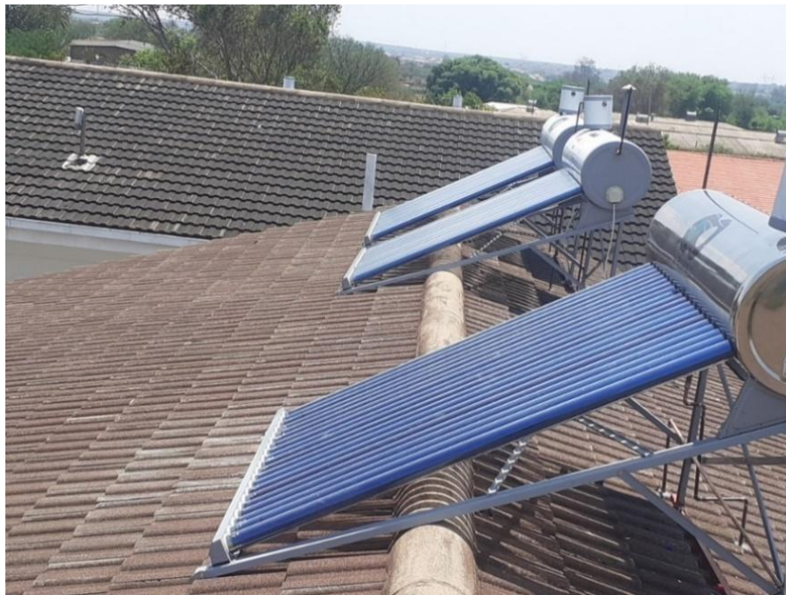
Figure 20. Thermosyphon system “CPS Sisters Convent of Lady Kingsdale”, view from south. Source: National University of Science and Technology (NUST), Zimbabwe.
