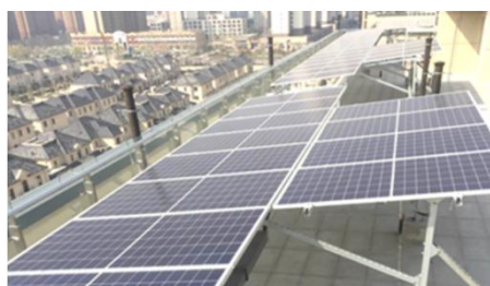
PV hot water integrated subsystem project in Cangzhou, Hebei Province
