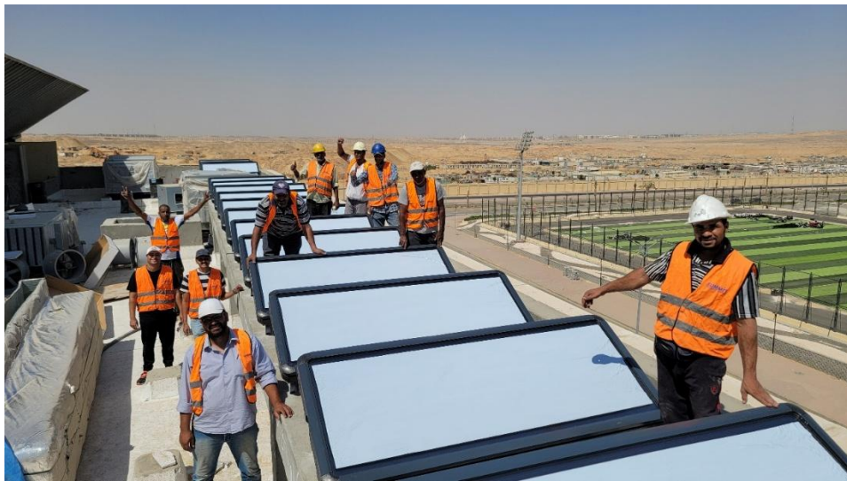
Figure 15. Collectors mounted on concrete skeleton to avoid shadowing Photo: Summit powered by GREENoneTEC
