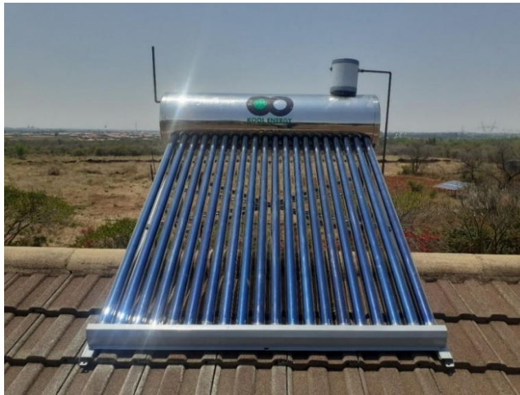
Figure 21. Thermosyphon system “CPS Sisters Convent of Lady Kingsdale”, view from north. Source: National University of Science and Technology (NUST), Zimbabwe.
